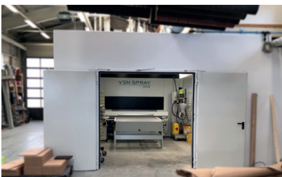
On-site spatial situation ideally solved: Machine was fitted in the room by means of drywalls
